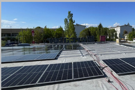
Solar power plant: 70 kWp / 60 kW
