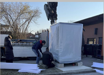
Battery storage system: 100 kW / 233 kWh
